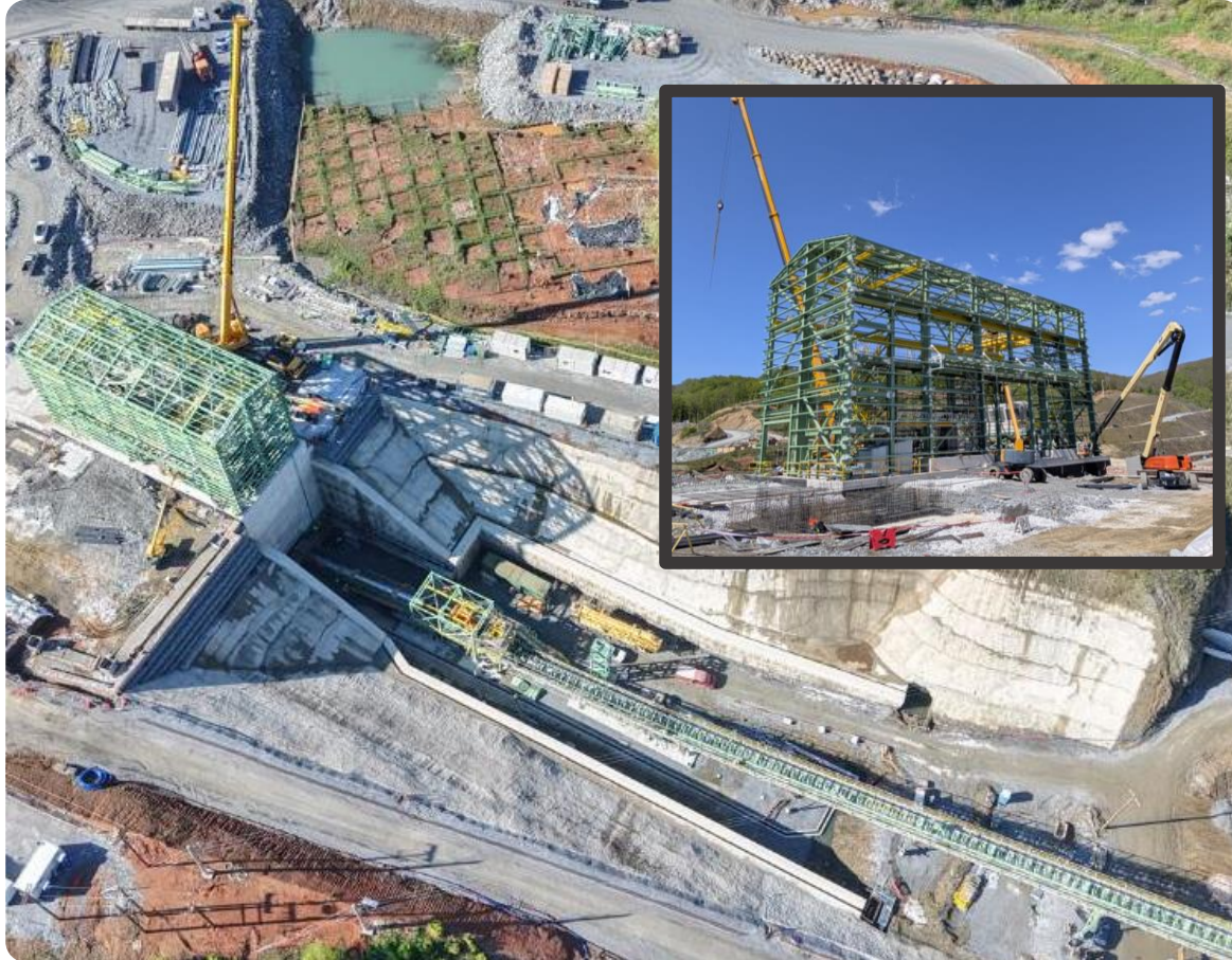
Primary crusher overview. Top right insert – closer up view of primary crusher building erection.
