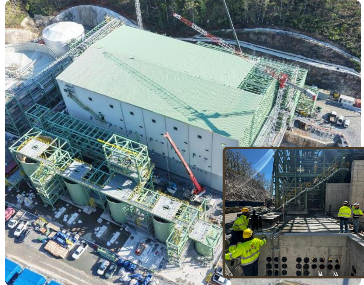
Tailings filter press building. Bottom right insert – closer up view of filter building pull pits.
